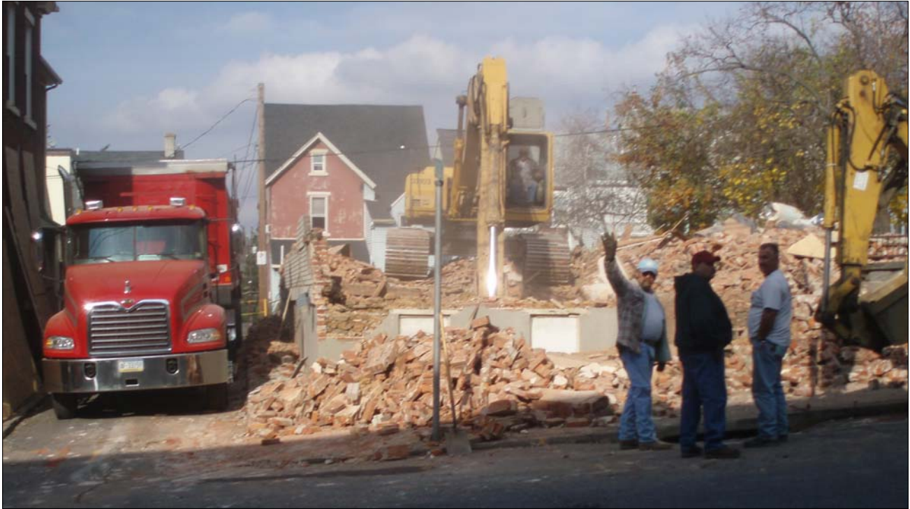
Above, photograph taken after demolition in preparation for Moravian IV. Photograph courtesy of Henry Hendricks.
